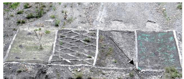
(b) 放水冲刷中边坡现状
