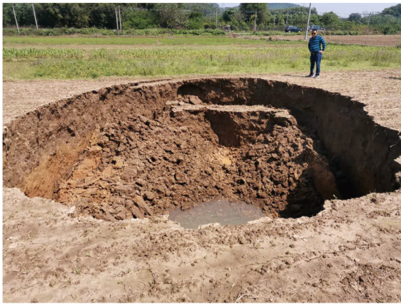
(a) T1塌陷坑
