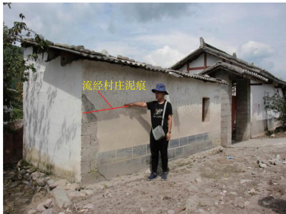
图 5 流经村庄泥痕 Fig. 5 Mud mark in the village
