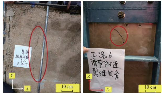
(a) 坡顶横向贯通裂缝
