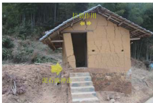
图 9 房屋变形破坏特征 Fig. 9 Deformation and failure characteristics of building
