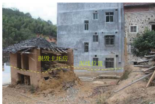
图 10 破坏房屋与淤积泥线 Fig. 10 Destruction of houses and siltation mud line
